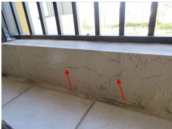
Photo #1 – Unit 208 crack in northeast knee wall.
