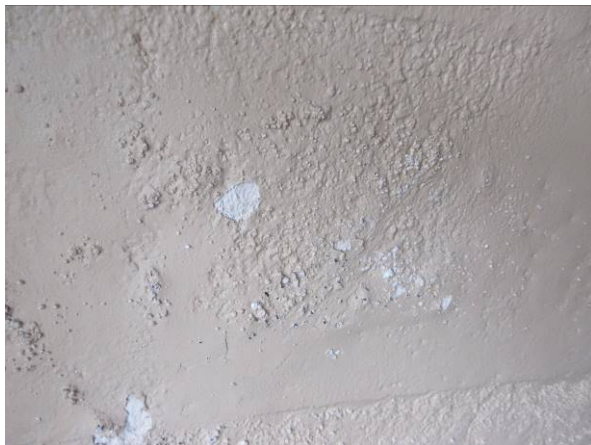
Photo #48 – North garage - evidence of peeling paint on the wall near the west entrance.
