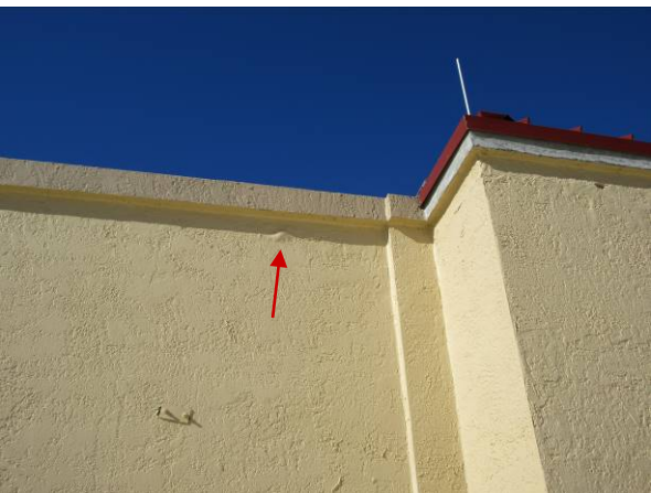
Photo #30 – Roof – blister in paint.
