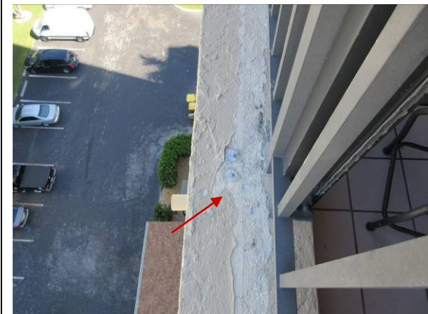
Photo #15 – Unit 908 typical damage to coating on the knee wall.
