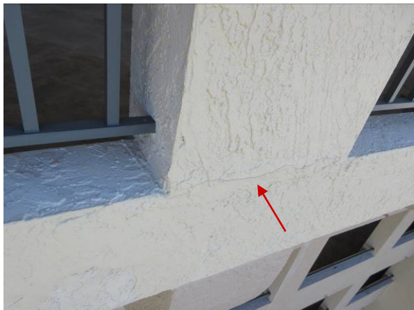
Photo #35 – Exterior walkways – typical hairline cracks in the stucco.
