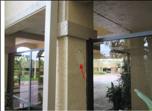
Photo #61 – Front of tower – peeling paint on column.
