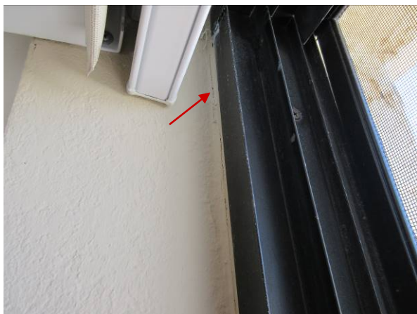
Photo #18 – Unit 1007 master bedroom window frame separation on the left-hand side.
