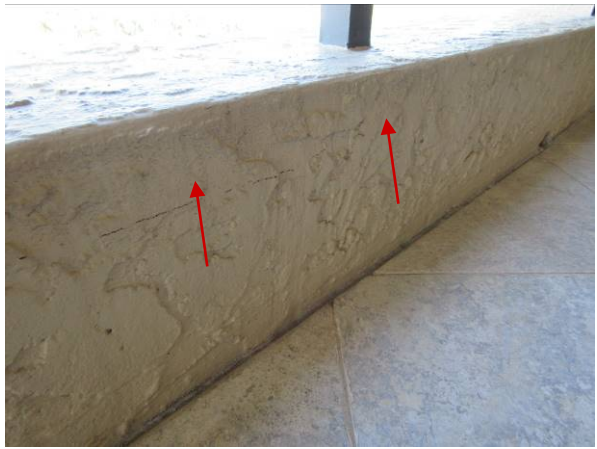
Photo #21 – Unit 1208 crack in north knee wall.
