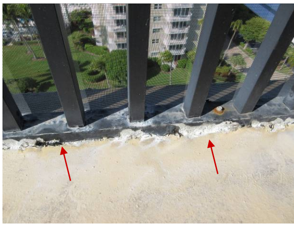
Photo #20 – Unit 1208 damaged aluminum screen enclosure.
