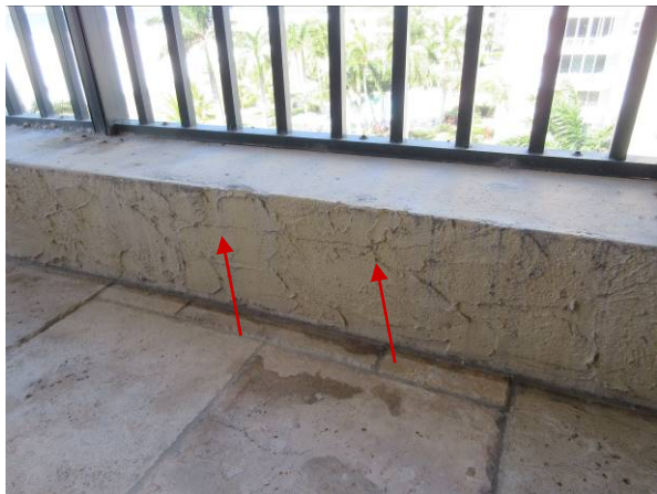
Photo #5 – Unit 608 crack in northeast knee wall.
