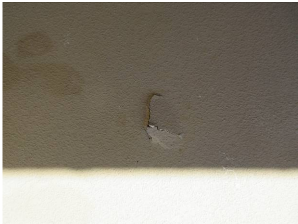
Photo #4 – Unit 604 spalled concrete.
