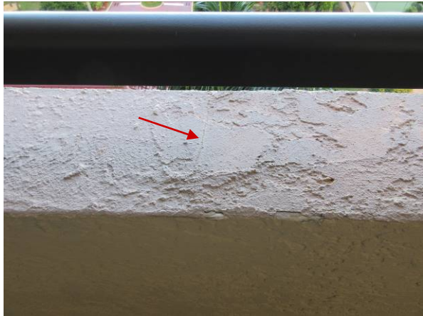
Photo #33 – Exterior walkways – typical hairline cracks on the knee walls.
