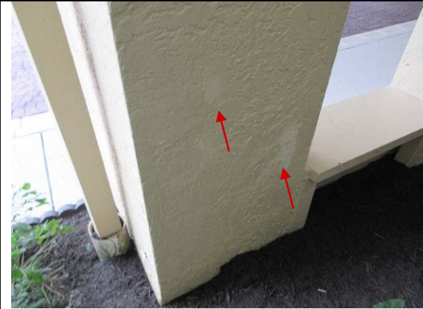
Photo #62 – Front of tower – peeling paint on column.
