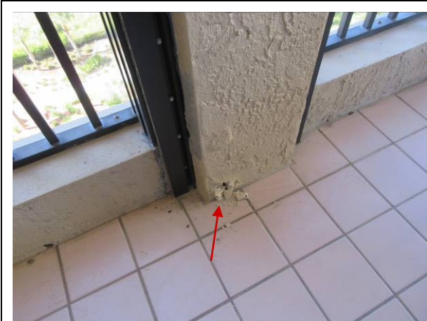
Photo #13 – Unit 908 damage to west column.
