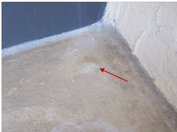
Photo #9 – Unit 801 blister in waterproofing in south corner
