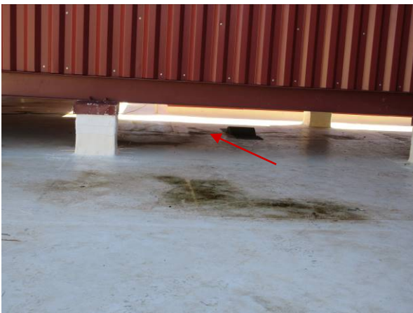
Photo #29 – Roof – Evidence of ponding water.
