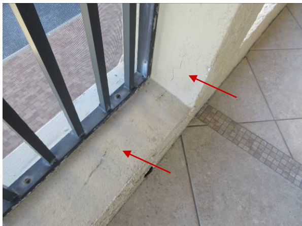
Photo #2 – Unit 308 crack in north knee wall and column.
