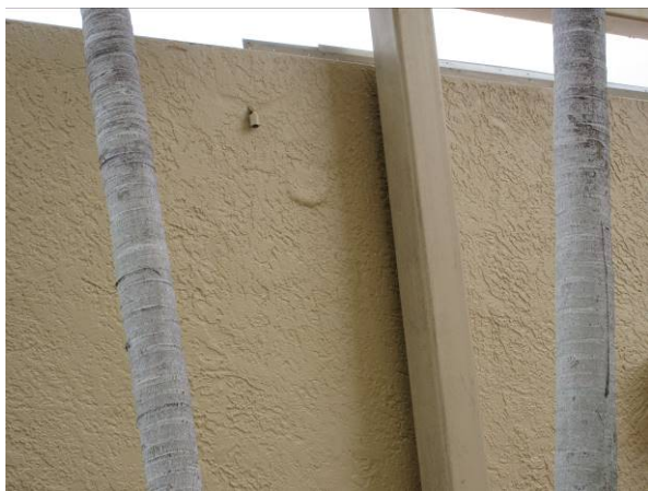
Photo #54 – South garage – blisters in paint near west entrance.
