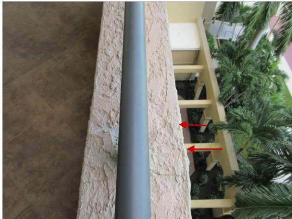
Photo #38 – Exterior walkways – potential concrete damage in front of unit 605.
