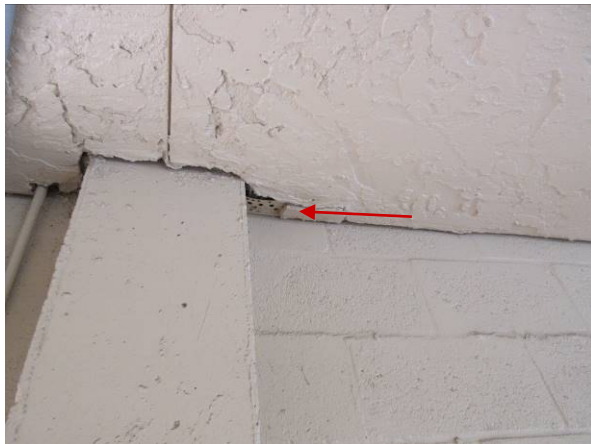
Photo #46 – North garage – damaged stucco near west entrance
