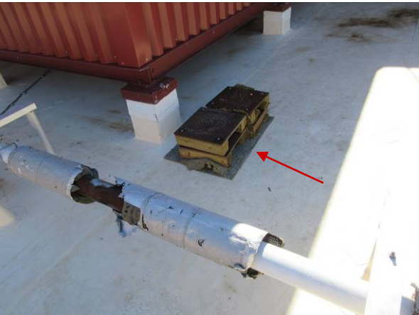
Photo #26 – Roof – typical loose debris.
