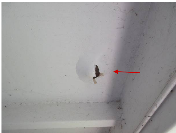
Photo #51 – South garage – blister full of water on the southeast corner.
