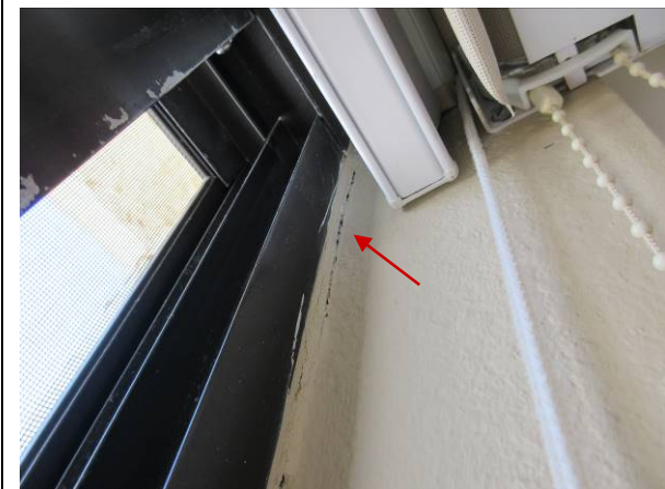
Photo #17 – Unit 1007 master bedroom window frame separation on the right-hand side.
