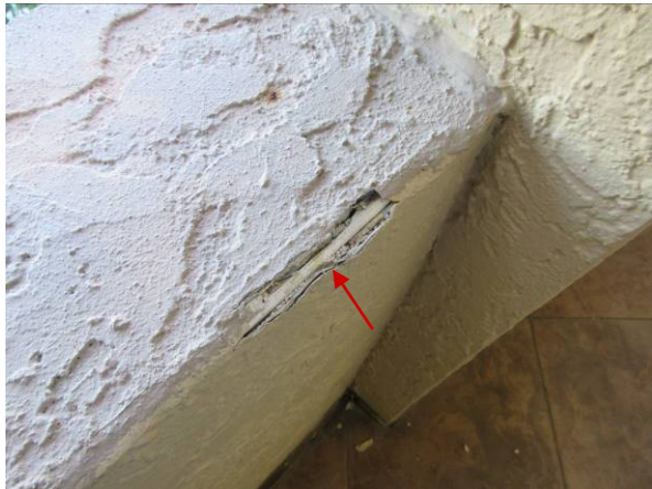
Photo #37 – Exterior walkways – damaged stucco in front of unit 703.
