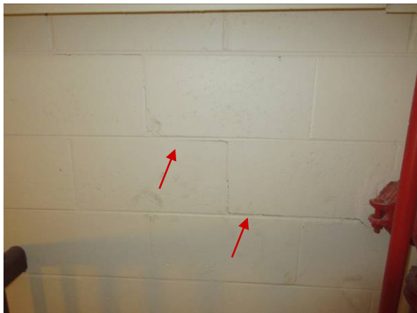
Photo #41 – South stairwell – stairstep crack on the roof level.
