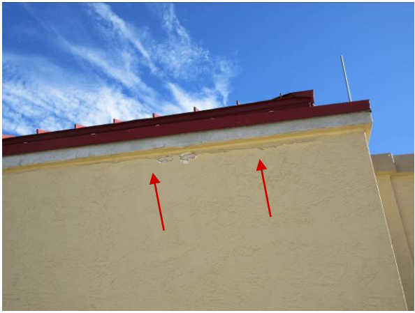
Photo #32 – Roof – cracked stucco on the elevator tower.
