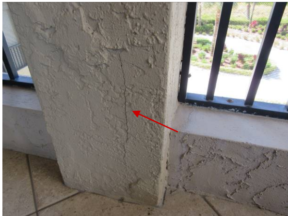
Photo #3 – Unit 308 crack in west column.
