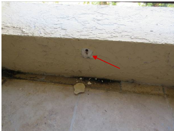
Photo #6 – Unit 608 exposed rust spot on north knee wall.
