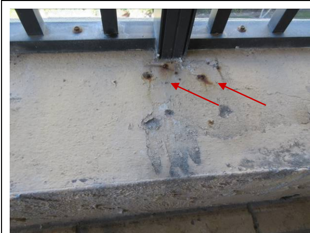
Photo #7 – Unit 608 rusted fasteners from old shutters.
