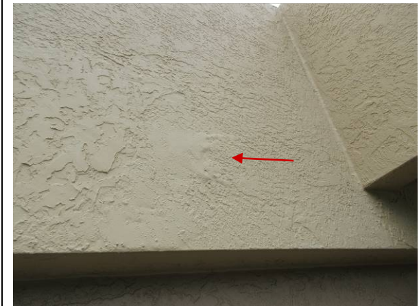
Photo #57 – South garage – blisters in the paint near the east entrance.
