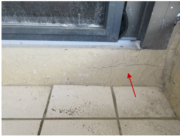
Photo #22 – TH-2 crack in the concrete below the sliding glass door on the 2 nd floor.
