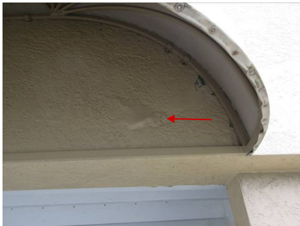
Photo #58 – South garage – blisters in the paint near the east entrance.
