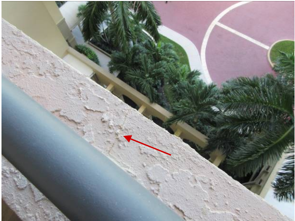
Photo #34 – Exterior walkways – typical hairline cracks on the knee walls.
