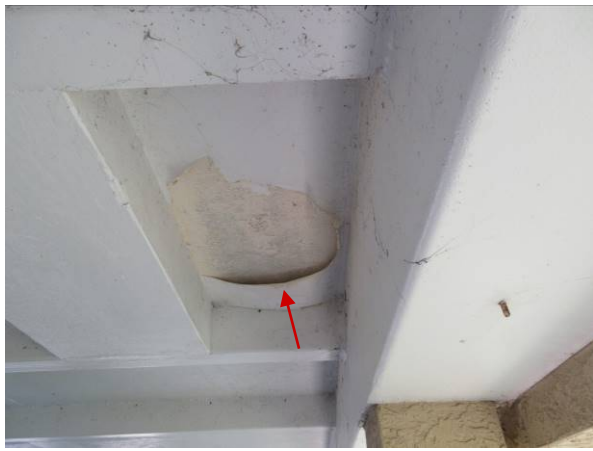
Photo #50 – South garage – peeling paint near the west entrance.
