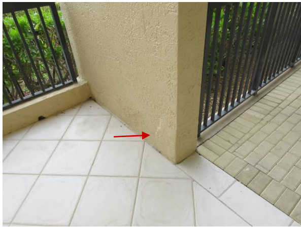
Photo #60 – Rear of tower – potential damaged concrete at base of the column outside common area entrance.
