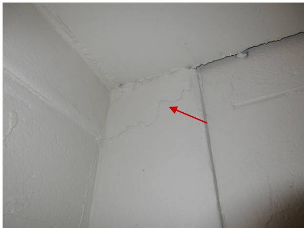
Photo #42 – North stairwell – potential concrete damage on the column between the 10 th and 11 th floor.
