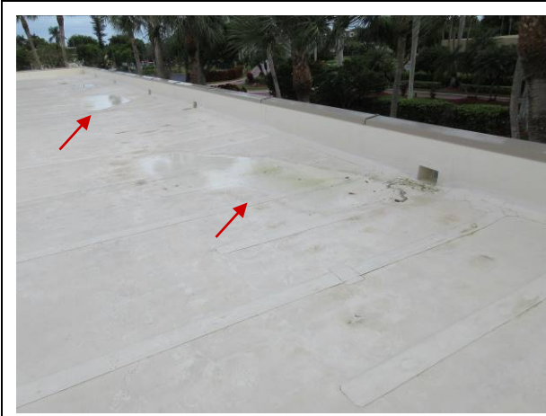
Photo #49 – North garage – evidence of ponding water.
