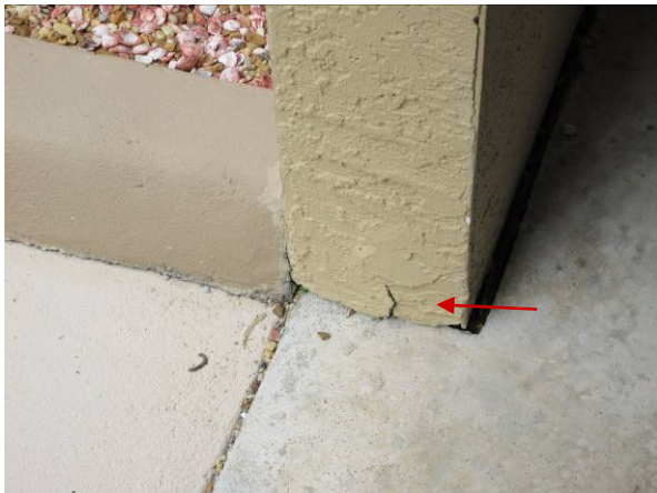
Photo #45 – North garage – crack in stucco at west entrance.
