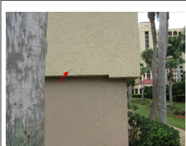
Photo #55 – South garage – peeling paint on the east end.
