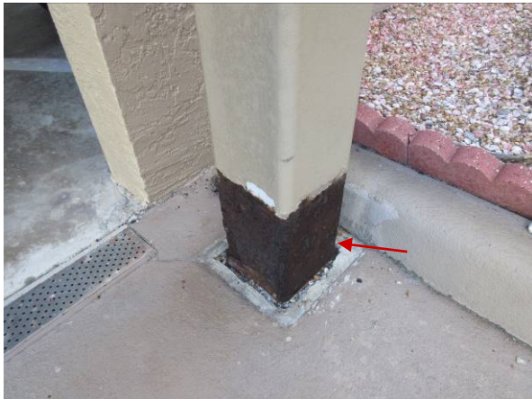
Photo #43 – Front awnings – typical base posts are rusted.
