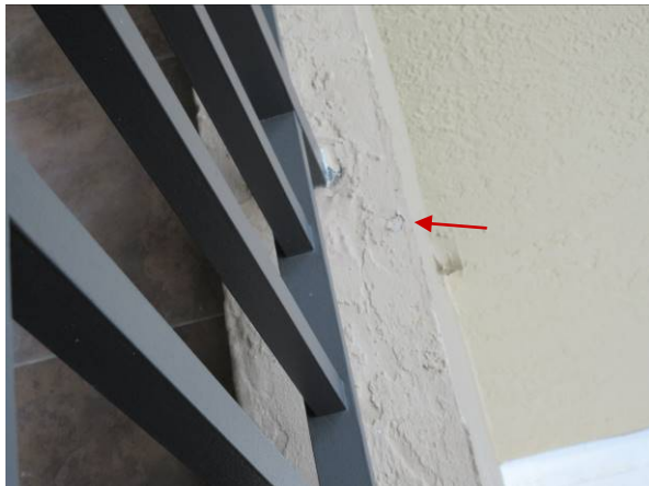
Photo #39 – Exterior Walkways – peeling paint on knee wall on balcony near elevators.
