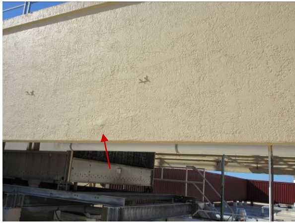
Photo #31 – Roof – blister in paint.
