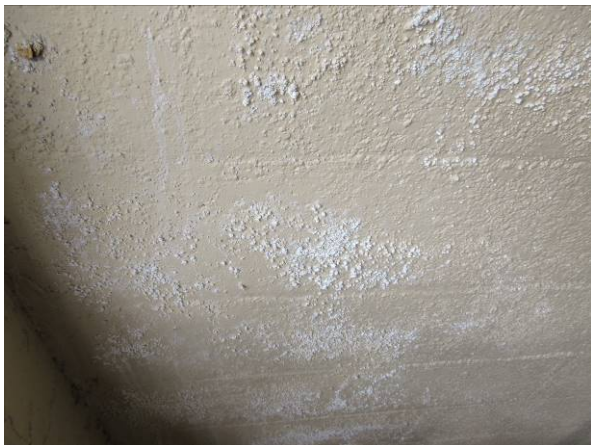
Photo #47 – North garage – evidence of efflorescence on the wall near the west entrance.
