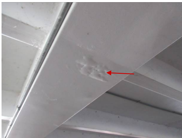
Photo #53 – South garage – blisters in paint on the south end.
