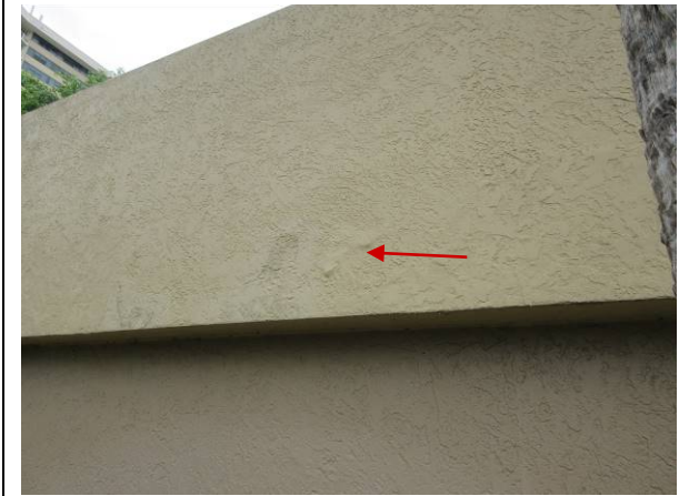
Photo #59 – South garage – blisters in paint on the southeast corner.
