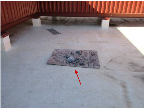
Photo #25 – Roof – typical loose debris.
