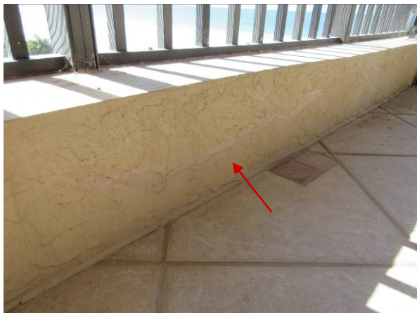
Photo #10 – Unit 800 crack in south knee wall.
