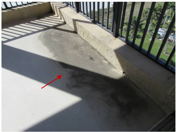
Photo #23 – PH-8 evidence of poor drainage.
