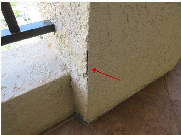
Photo #36 – Exterior walkways – damaged stucco on column south end on PH level.
