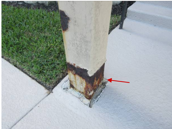
Photo #44 – Front awnings – typical base posts are rusted.
