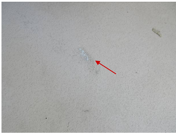
Photo #24 – PH-8 damage to the waterproofing.
