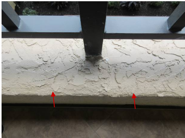
Photo #40 – Exterior walkways – potential concrete damage in front of unit 206.
