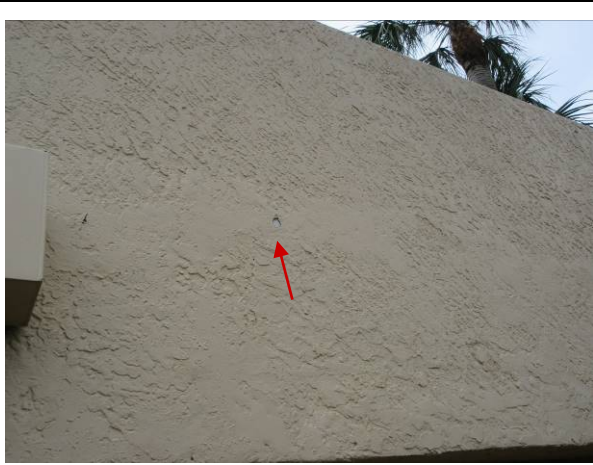
Photo #56 – South garage – hole in the stucco near the east entrance.
