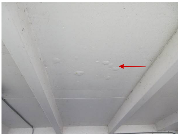
Photo #52 – South garage – blisters in paint on the south end.
