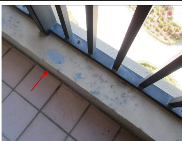
Photo #14 – Unit 908 typical damage to coating on the knee wall.
