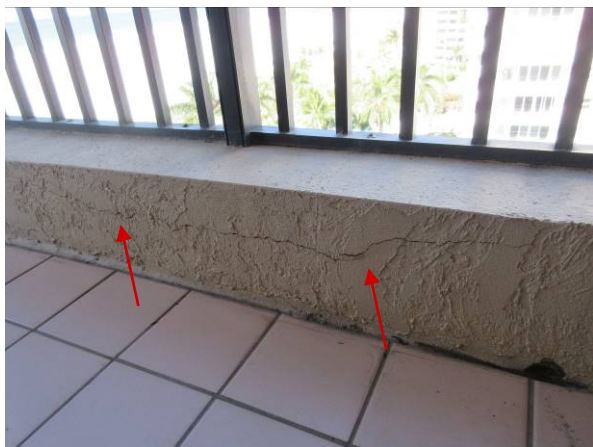
Photo #12 – Unit 908 crack in northwest knee wall
