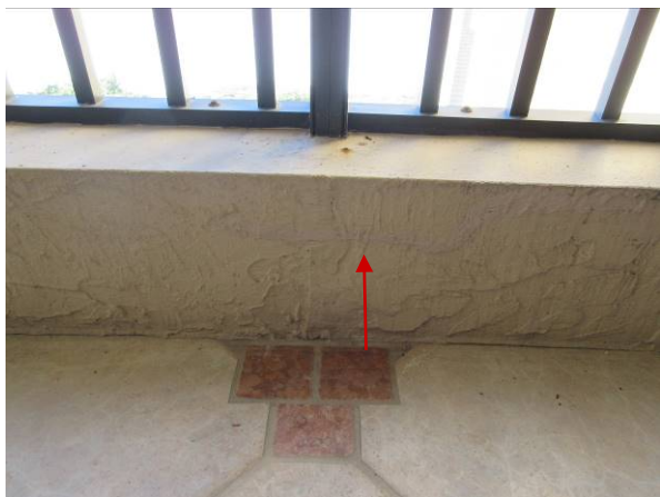
Photo #11 – Unit 800 crack in west knee wall.
