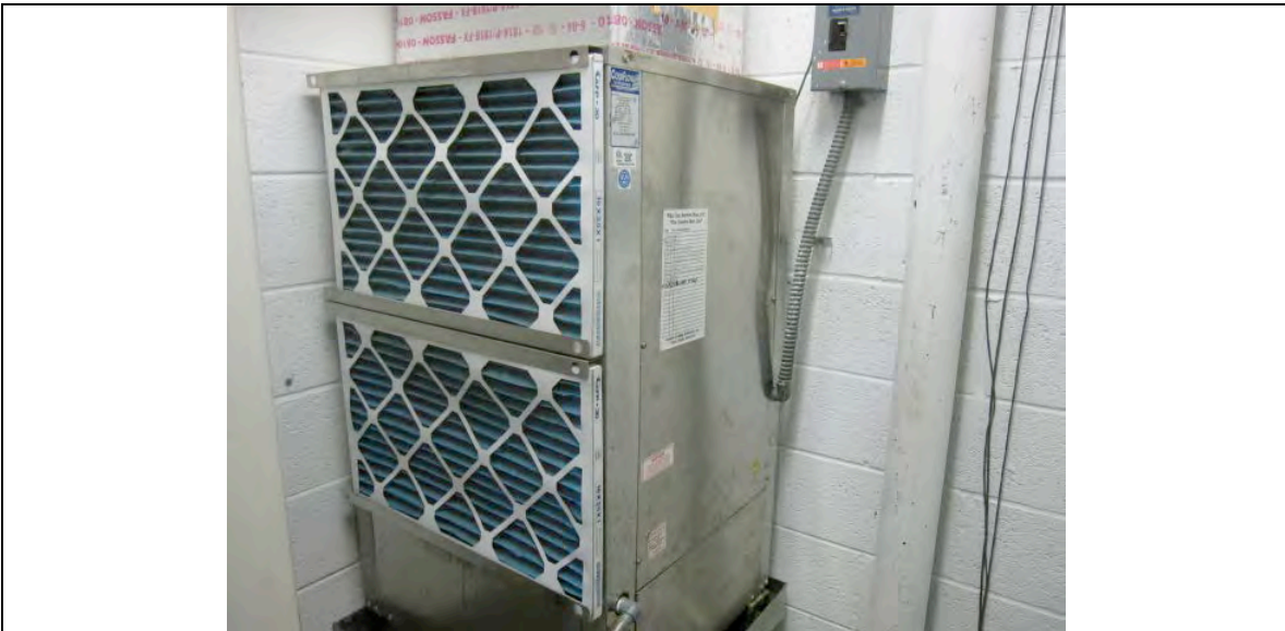
AC Equipment, Social Room
