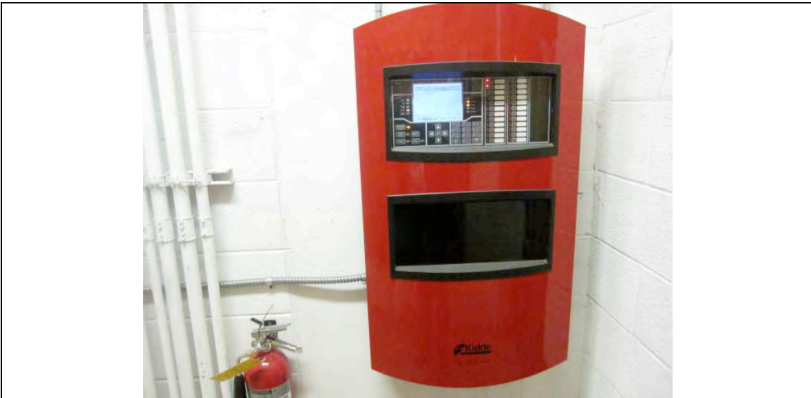
Fire Alarm Control Panel
