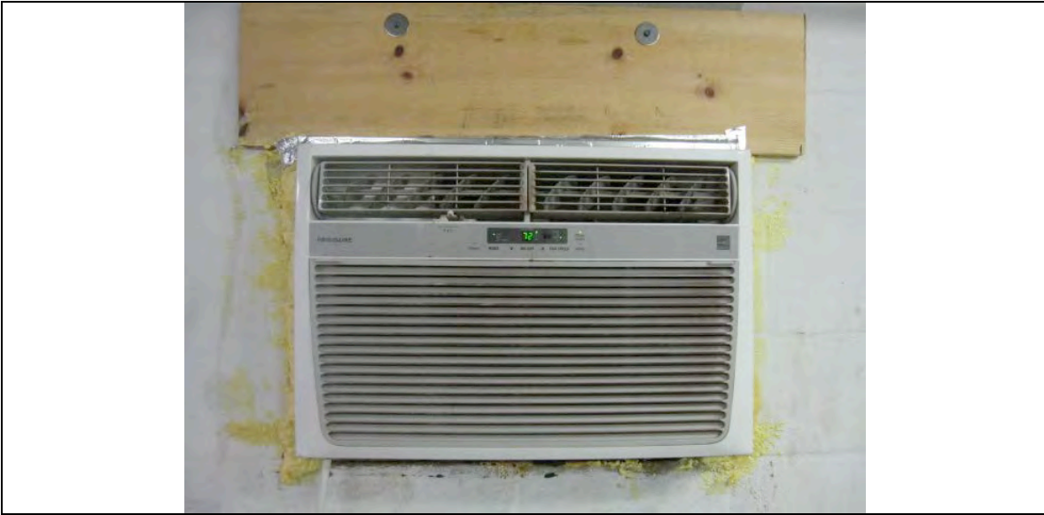
AC Equipment, Elevator Room
