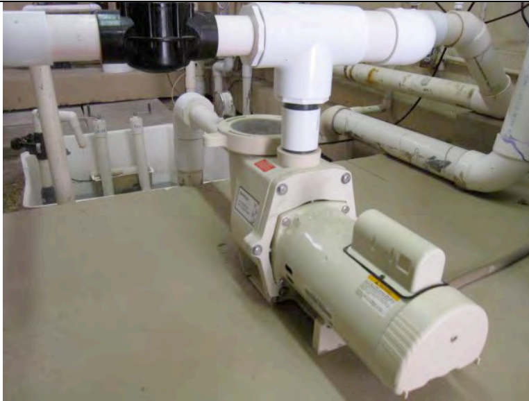
Pool & Spa Equipment
