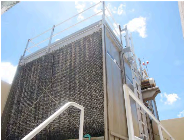
AC Cooling Tower
