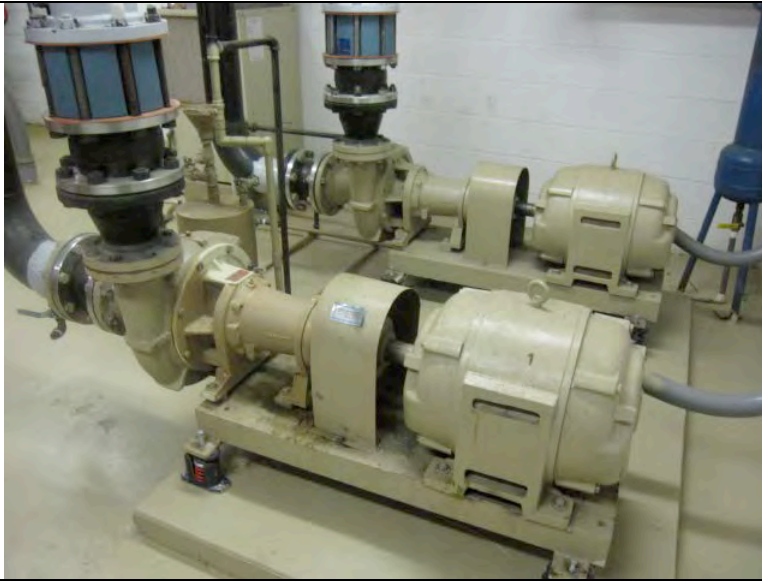
AC Circulating Pumps
